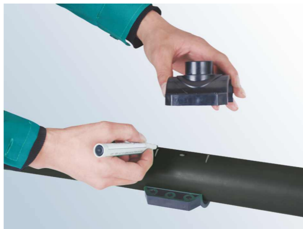
4. Use a marker to draw a reference line on the pipe to allow reinstalling the saddle, unscrew the nuts and remove the saddle.
