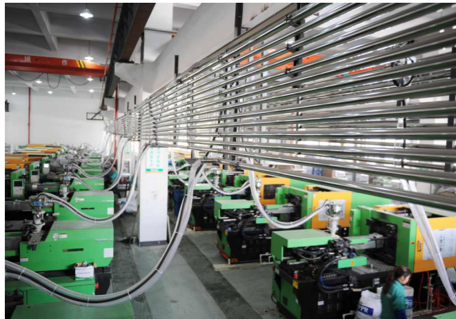
Automatic Feeding System
